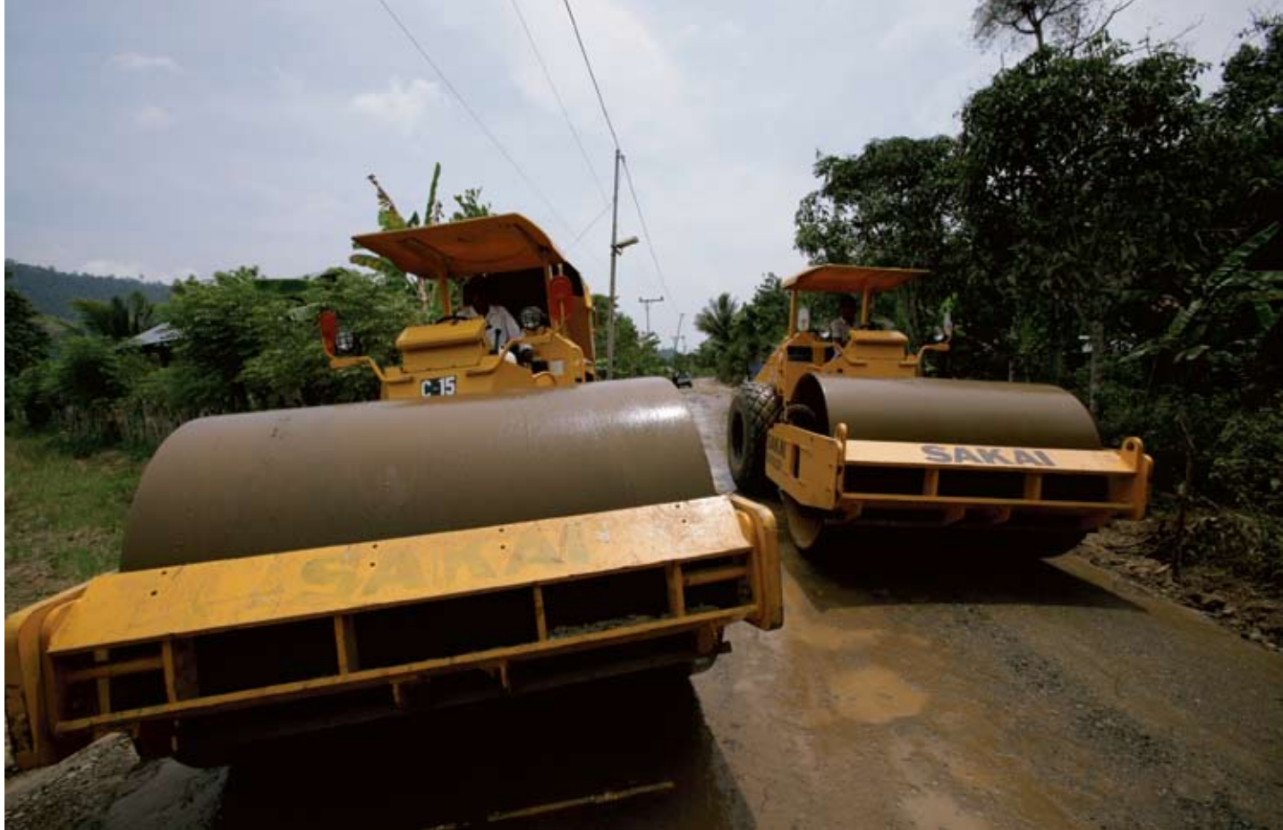
Heavy equipment for pressing a road built by USAID in Lamno, Aceh Jaya, March 18, 2006. Photo: BRR/Arif Ariadi
